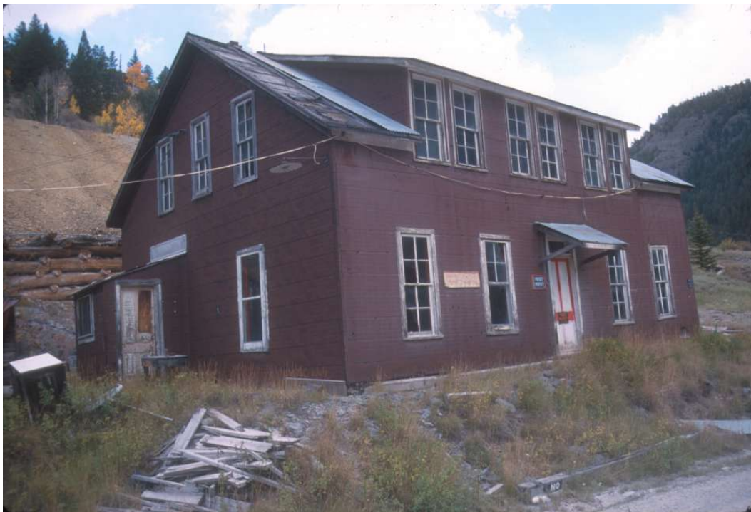
HP 17. 2001 photo of the southwestern and northwestern sides of the boarding house (Building 16), looking east-southeast. Note the original windows and door in place.
