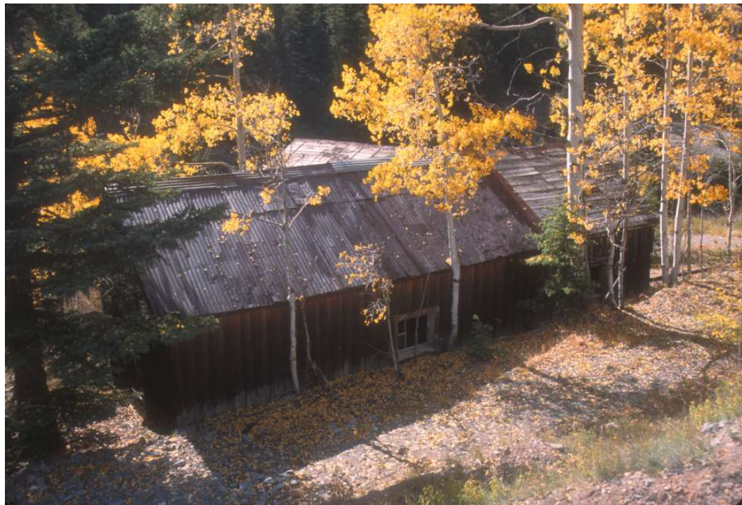
HP 10. 2001 photo of the northeastern side of the office (Building 9), looking west-northwest.
