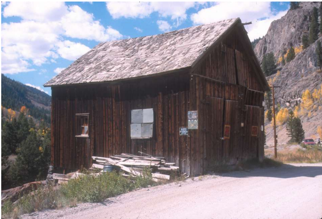
HP 21. 2001 photo of the southeastern and northeastern sides of Building 36, looking west. This building collapsed and was removed soon thereafter.
