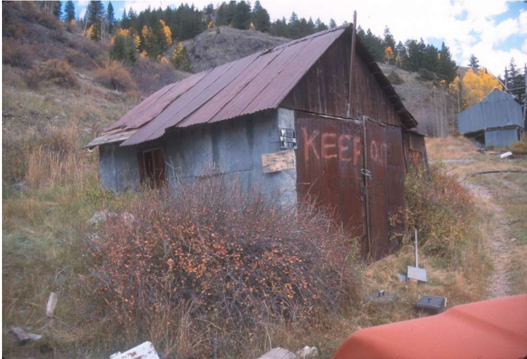
HP 24. 2001 photo of the southwestern and northwestern sides of Building 39, looking east. This building later collapsed and was removed.
