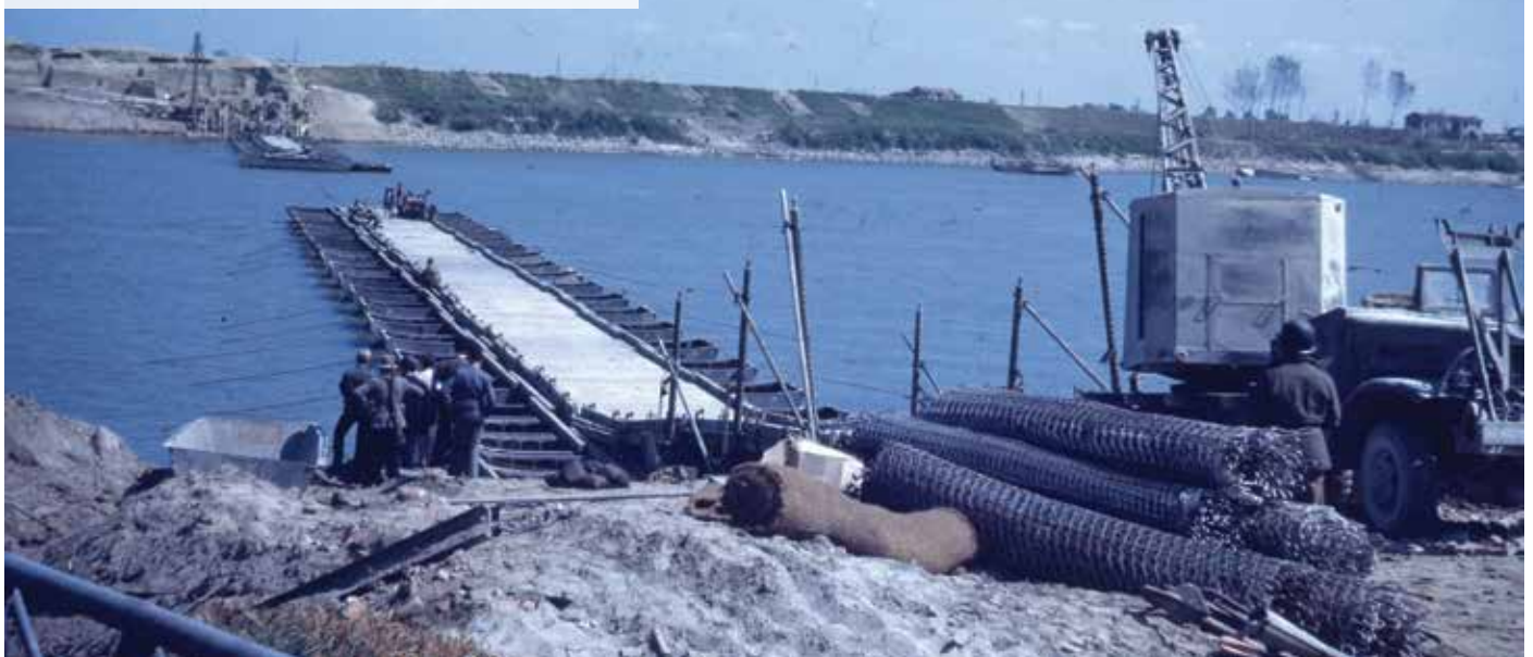
A pontoon bridge under construction which will carry the division across the Po River. History Colorado, 2020.44.51
