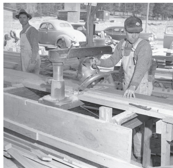
▼ A carpenter cuts a board to length. In order to meet the deadline, work went on six and sometimes seven days a week. Attention to detail and craftsmanship were important to Pando Constructors. Although the November 1942 deadline loomed, there is no indication that any shortcuts were taken by the builders. Courtesy of Denver Public Library
