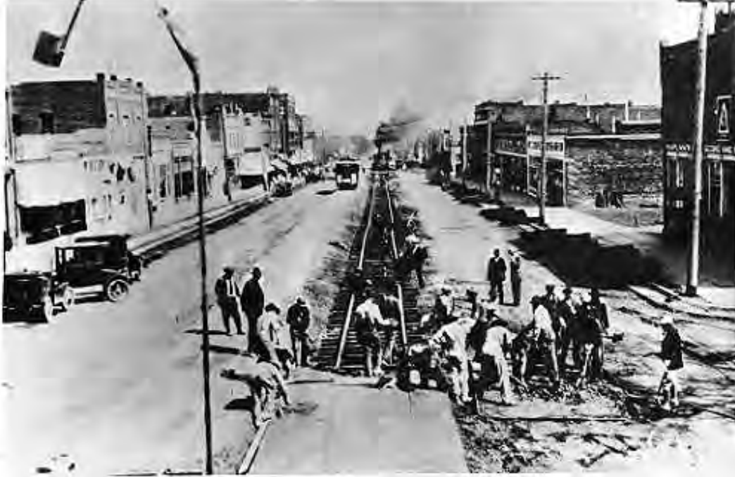
Figure 32. Construction of the streetcar tracks on Colorado Avenue in Colorado City, date unknown. 220
