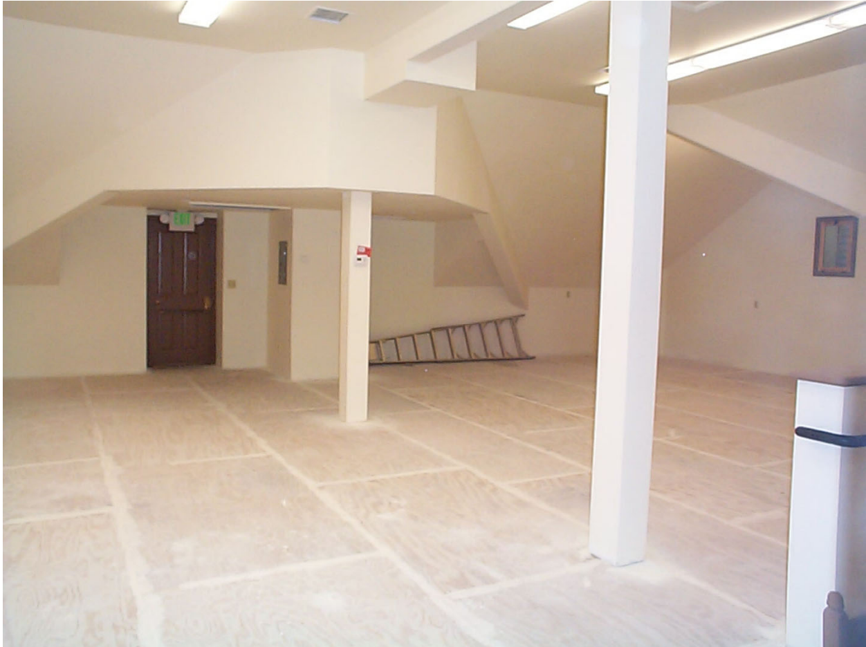
HP9. The Animas City School/ Animas Museum in 2008 inside the reconstructed roof/new Collections area. Camera looking northwest.
