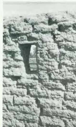
The WPA adobes with a higher percentage of pebbles than in the original.
